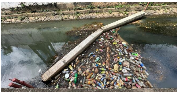
Figure 2: The waste being intercepted by the Ocean Strainer which installed at Dehimalwatte Canal
